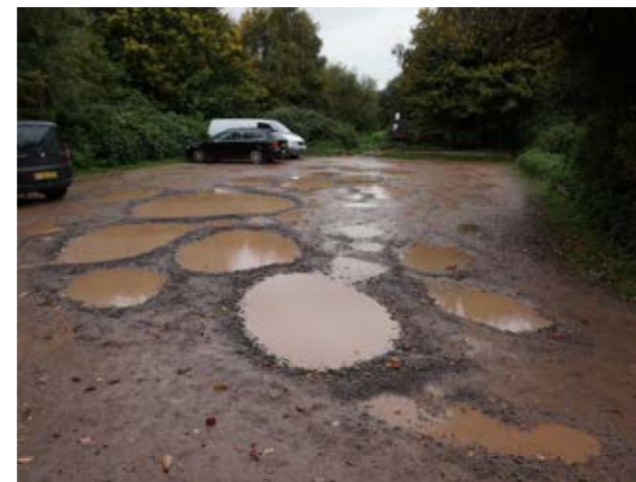
Photograph 13: Pot holes at Bersted Brooks LNR car park.
